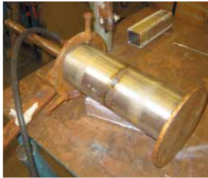
Back shielding: This stainless steel pipe has been set up or back shielding by using two cover plates at either end.
