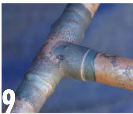
9 Once cool, the finished join should be inspected. Note there is no problem with quenching the fitting with water to cool it down; this only anneals the copper.
