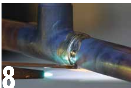
8 It should now be possible to brush the tip of the rod around the joint as it melts. The liquid solder will wick into the fitting, creating a neat join. There should be an even amount of solder around the circumference of the joint. You should be able to use the application of heat to draw the solder around the fitting.
