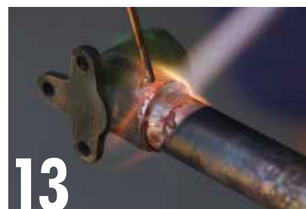
13 Soldering is much the same as with the copper fittings. Touch the tip of the rod to the fitting, and if it wets on contact, run solder into the joint until it travels the circumference of the fitting.
