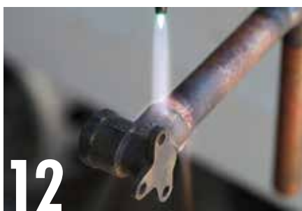
12 Heat the joint, concentrating the majority of the heat into the brass fitting. Once it reaches a dull red colour it should be ready for brazing. Note the flux, which has changed colour to dark red.
