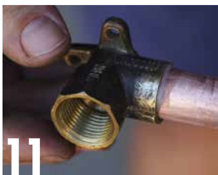
11 Insert the pipe into the fitting and give it a wiggle to distribute the flux.
